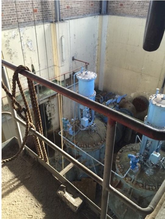
Figure 2.22: Interior, looking towards shafts, Valve House, 2015. Source: Dahua via City of Sydney
