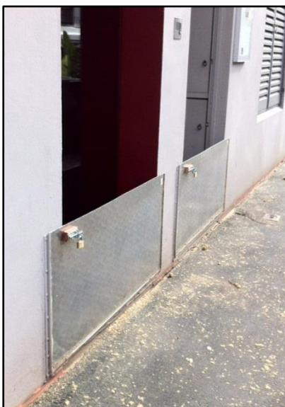
Photo 3: Flood gate at front door of residential property
