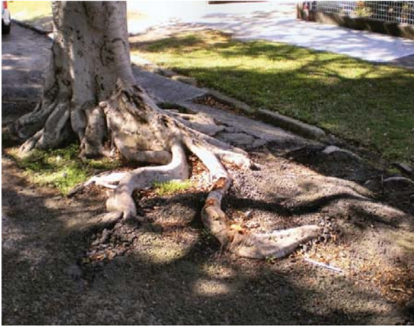
Photo 6: Existing kerb and guttering within Duke Street area is affected by tree roots.
