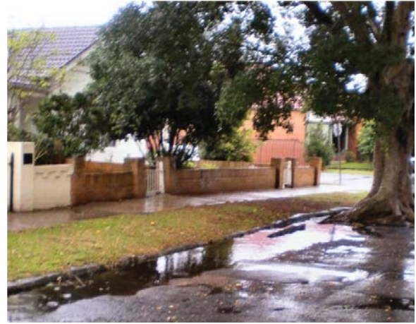
Photo 7: Localised ponding in Duke Street following minor rainfall.
