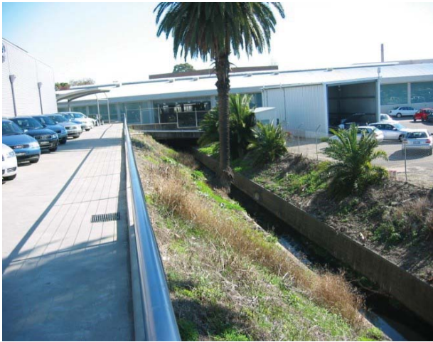
Photo 3: Sydney Water trunk drainage line from West Kensington.
