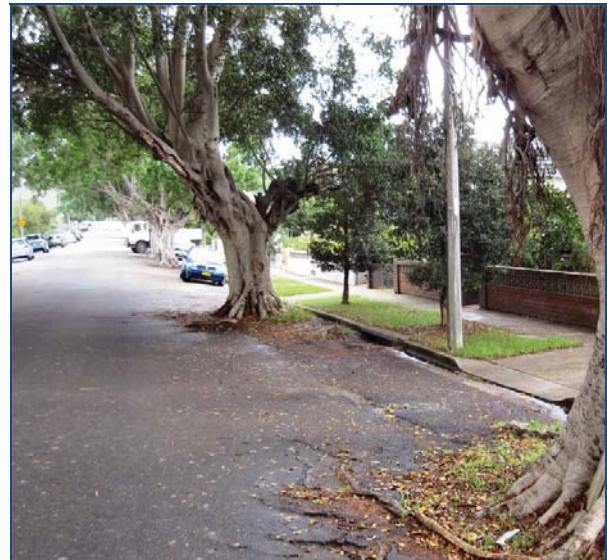
Photo B2: Trapped low point in Milroy Avenue.
