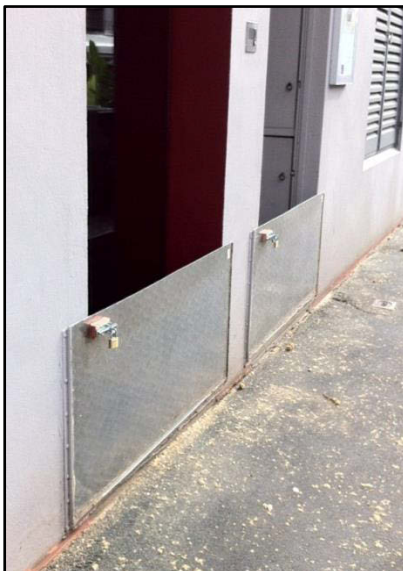
Photo 5: Flood gate at front door of residential property
