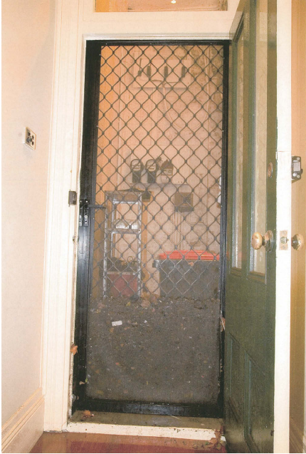
Floodmarks at residence entrance on Victoria St, Potts Point
