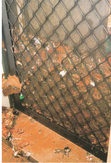
Floodmarks at residence entrance on Victoria St.
